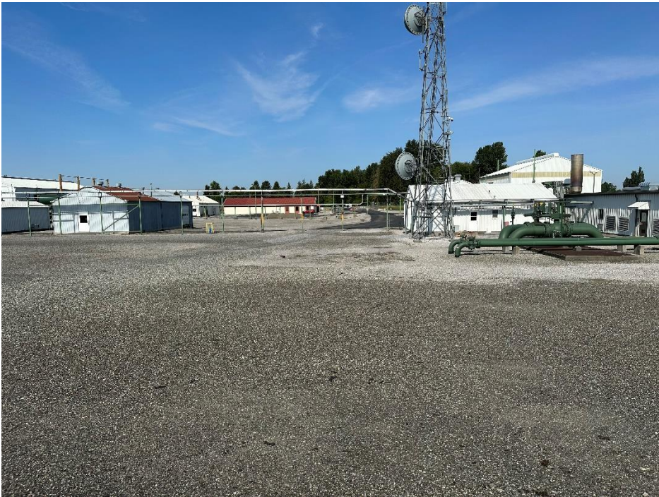
Photo 2. Compressor station infrastructure.
