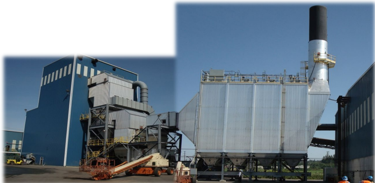
Figure 2-14 Boiler House and ESP
