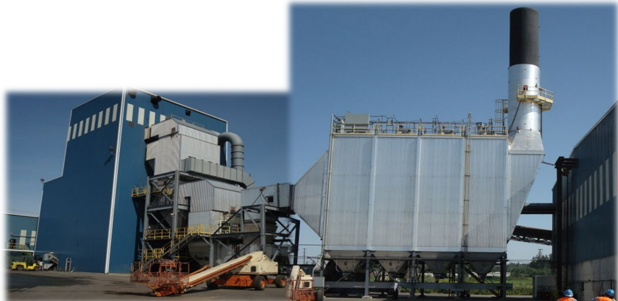
Figure 2-14 Boiler House and ESP
