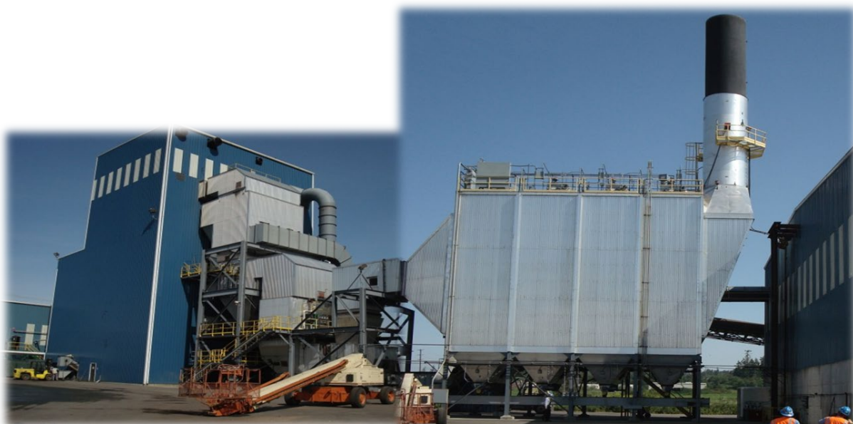
Figure 2-14 Boiler House and ESP
