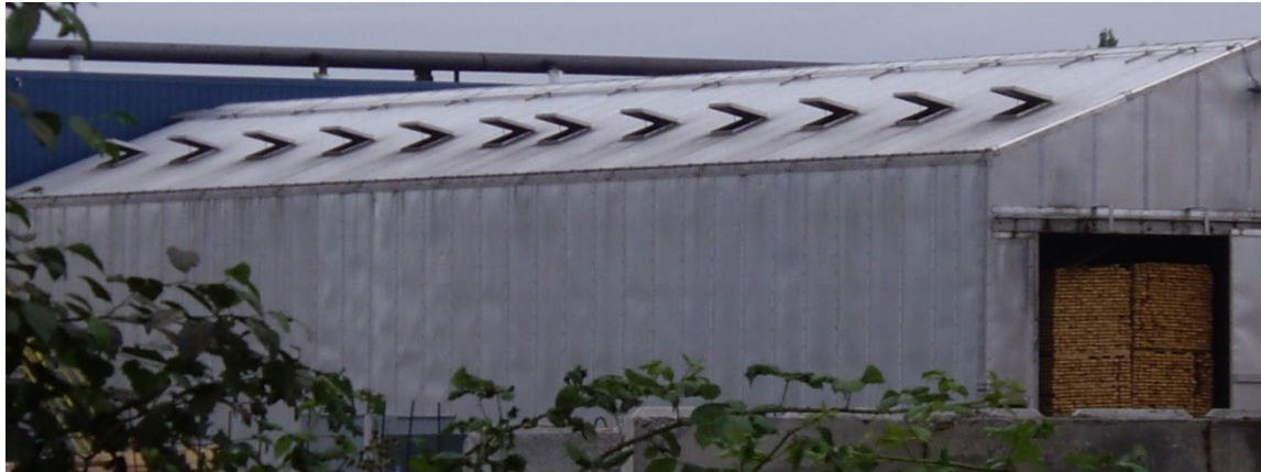
Figure 2-9 Dry Kiln at Cycle End
