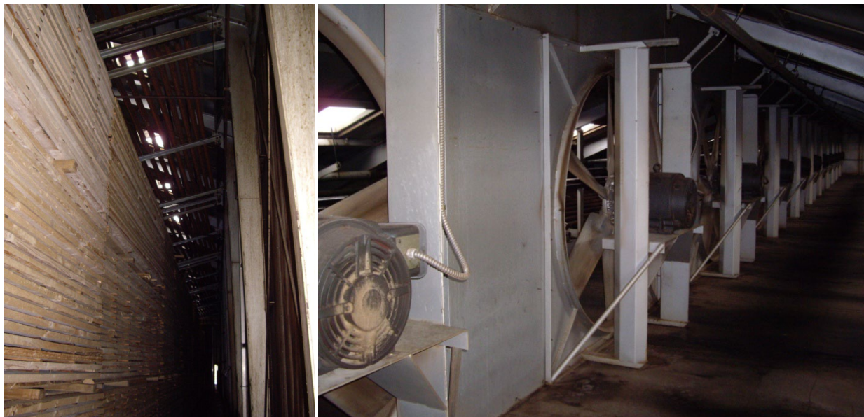
Figure 2-11 Kiln Internal Equipment
