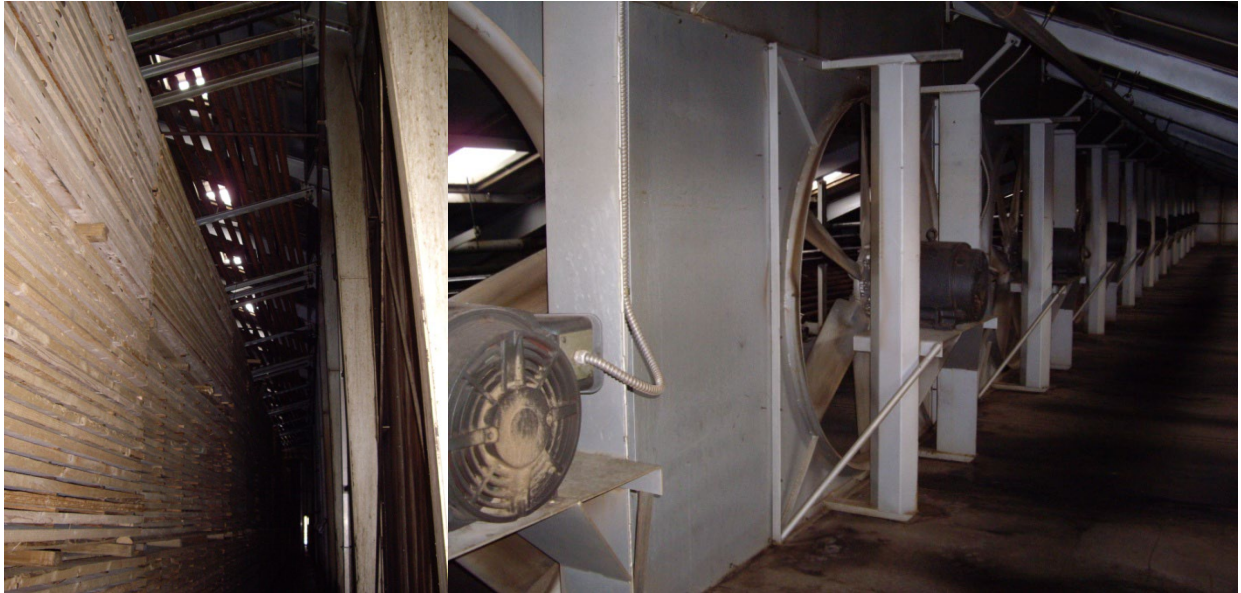
Figure 2-11 Kiln Internal Equipment
